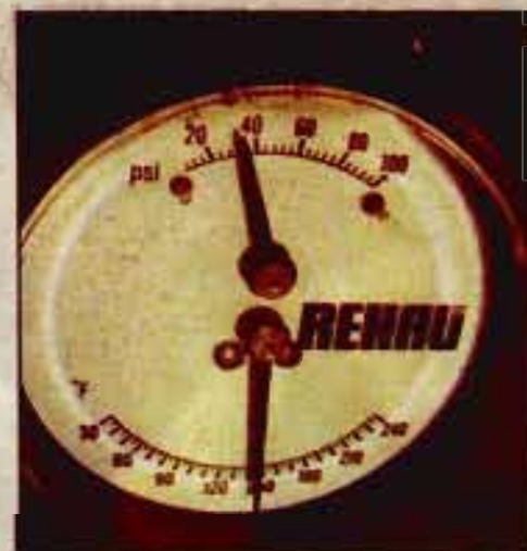
A gauge showing the water pressure and water temperature.
